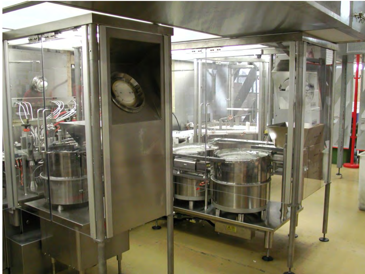
Barrier Fill Line Process
