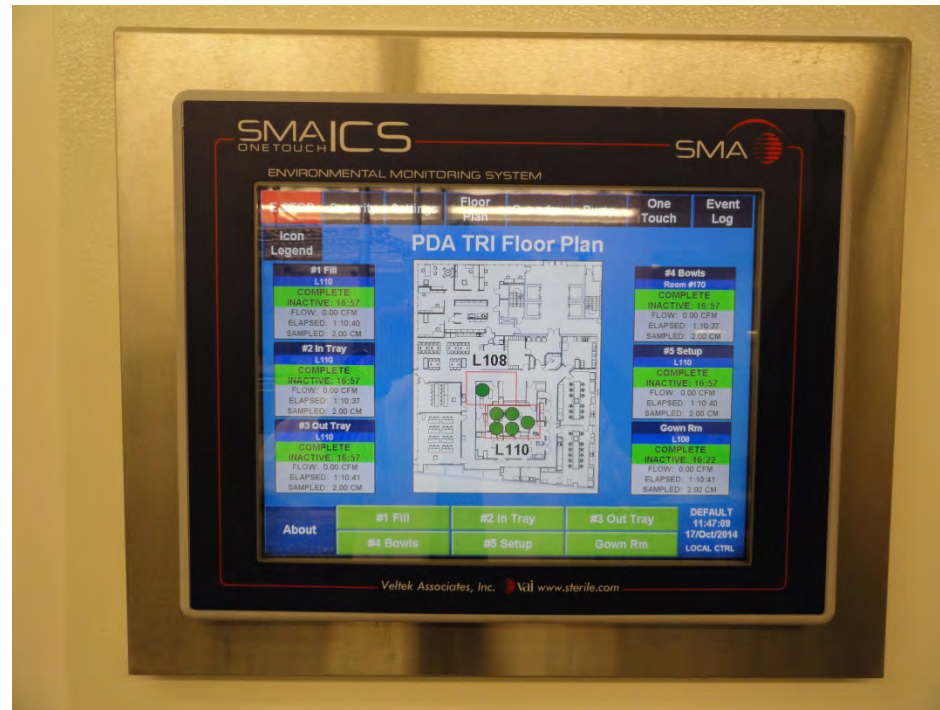
SMA Control Panel
