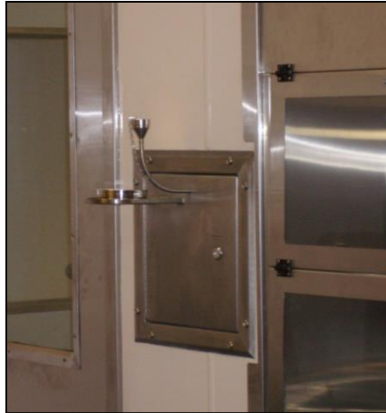
Flush mount (inside wall enclosure)
